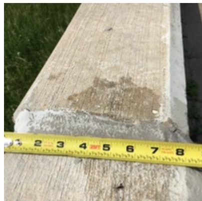
Caulk in abutment joint
