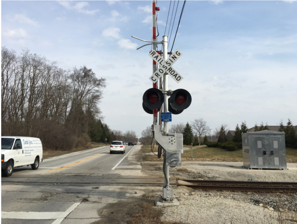
Photograph 11 Flashers & Gate (Facing North)
