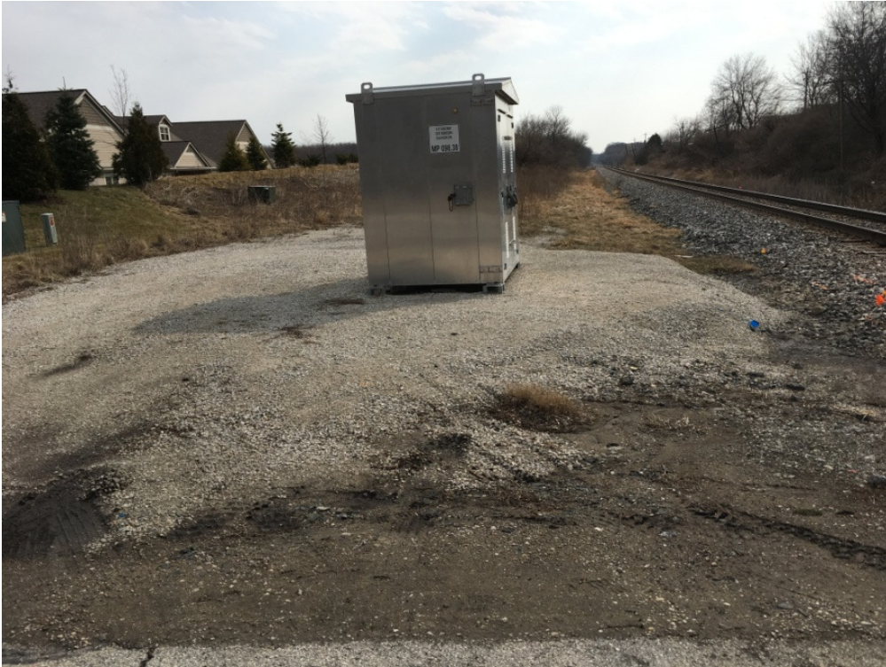
Photograph 9 Signal Cabinet (Facing East) Date: March 24, 2017
