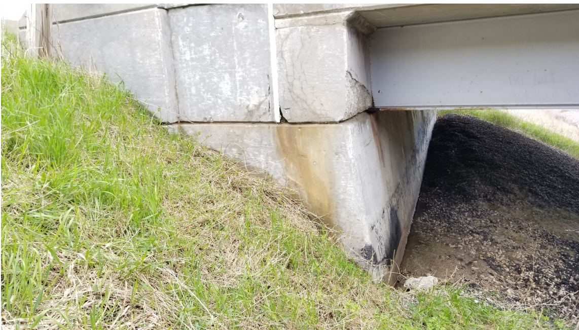
Concrete condition on NE abutment corner.
