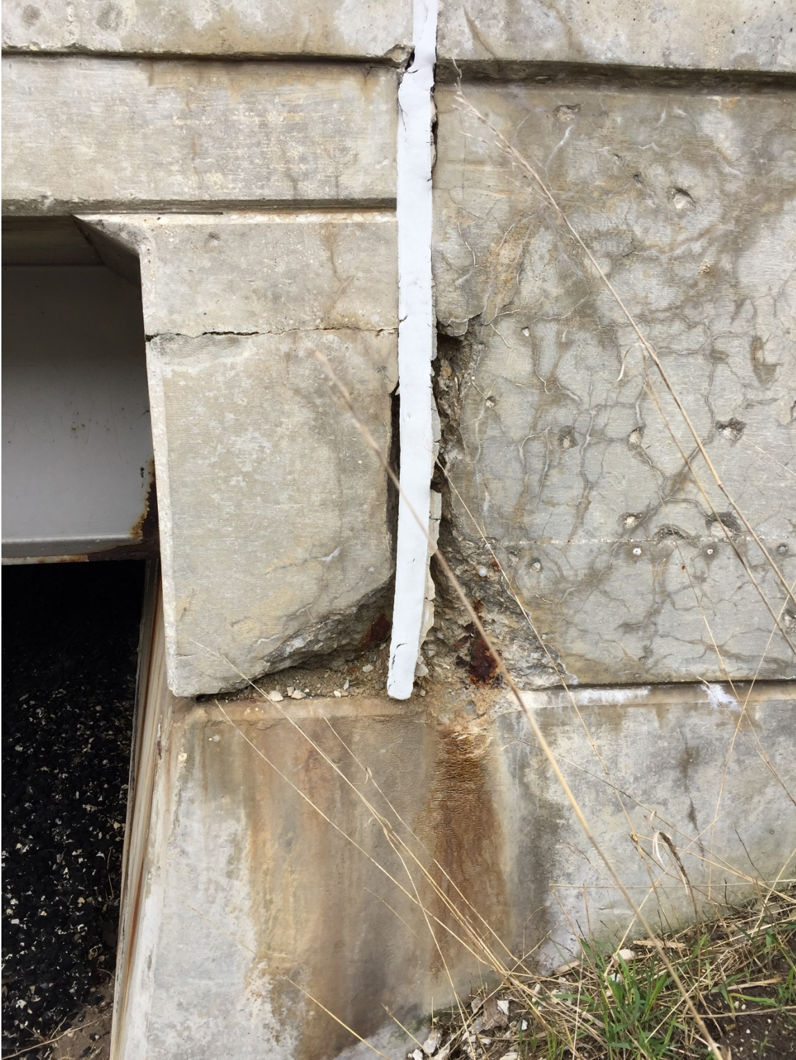
Concrete condition on SE abutment corner.
