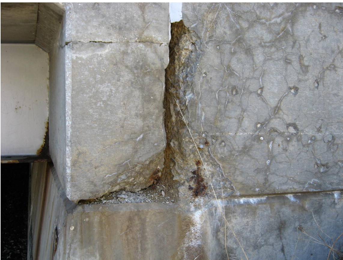
Concrete condition on NW abutment corner.
