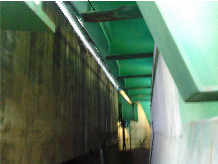
CLEAN AND PAINT THE APPROACH GIRDER BOTTOM FLANGES INSIDE THE BASCULE PIERS.
