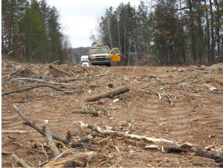
Town Road Condition After Logging Operations
