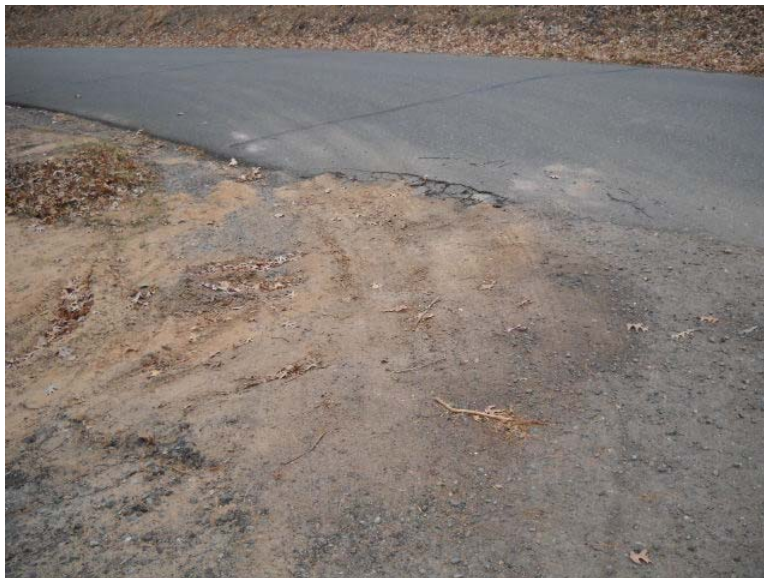
Road Damage from Logging Trucks
