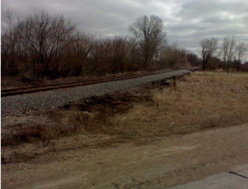
Photo #13 At Stop Clearing Sight Distance Right (North)
