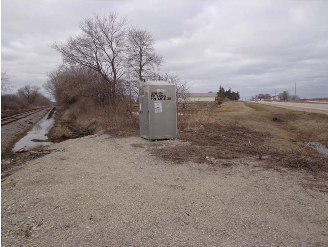
Photo #11 Signal Cabinet
