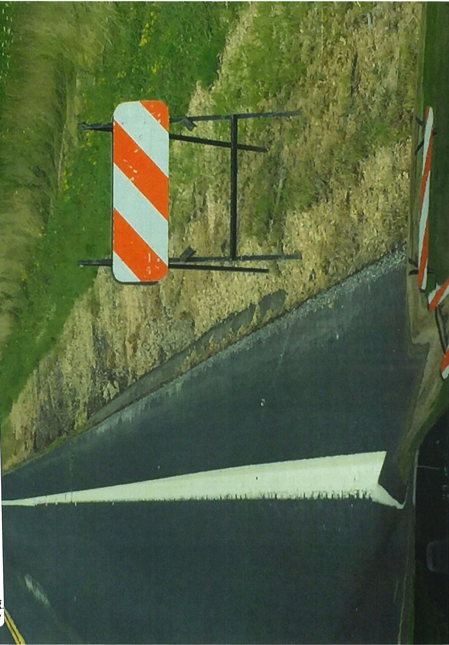
Hwy 95 Lakes Coulee Bridge Water over roadway
